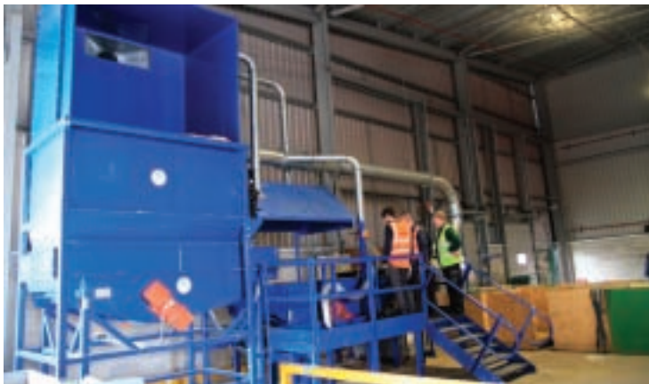
The sawdust separation plant installed at Pets at Home has doubled recycling rates at its National Distribution Centre
