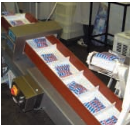
Straight from the bagger: Metal Detection installation at Whit Products in Tipton
