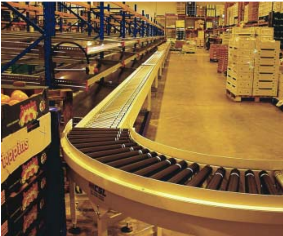
Eco-Box packing line: Conveyor Systems' installation for food distributor Pauleys, Corby
