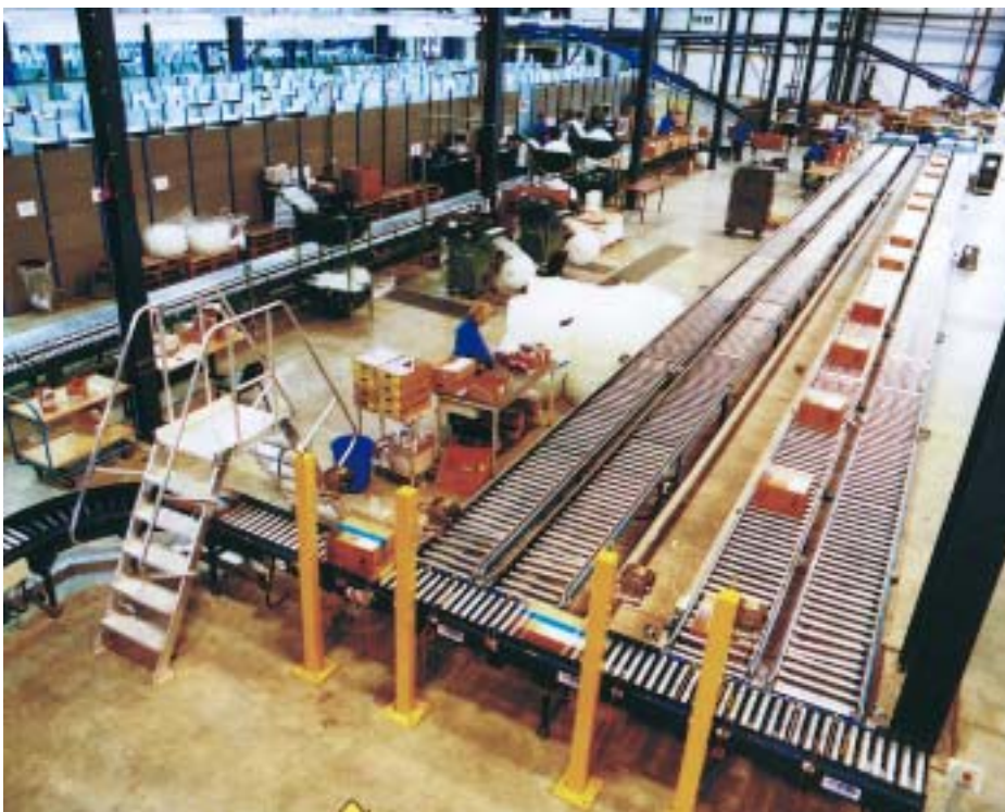
Pick and pack: CSL took just four weeks to install this 500 metre system for Universal Music Group
